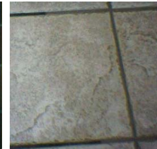
Grout w/ Severe Soil and Stains
