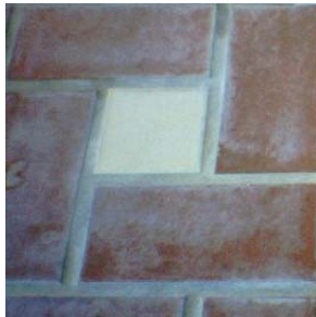
Pool Tile w/ Efflorescence
