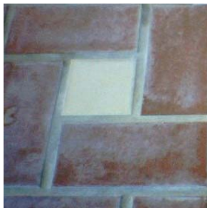
Pool Tile w/ Efflorescence
